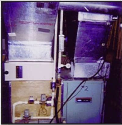
Heat Exchanger for the American Legion building
