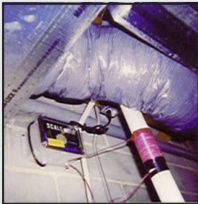
ScaleBlaster™ installed Spring, 1997
