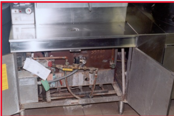
Base of steamer shows matter expelled after ScaleBlaster™ was installed.
